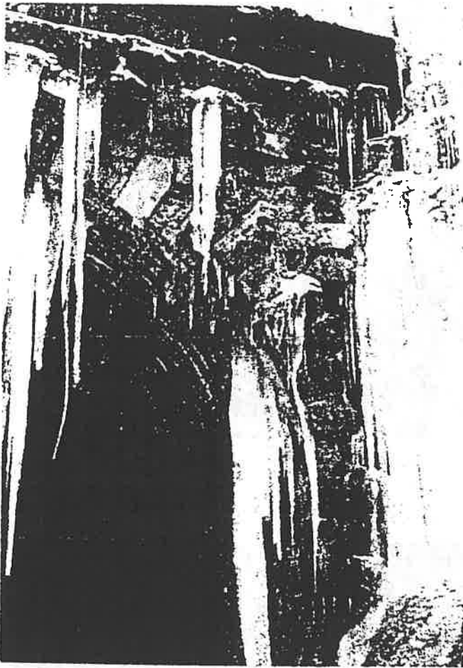
Photograph No. 3: Deteriorated Masonry at South Portal.
